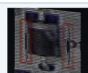
Jumper / link missing
